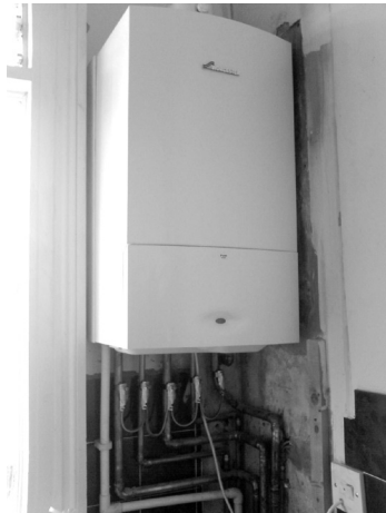
Caldera a gas
